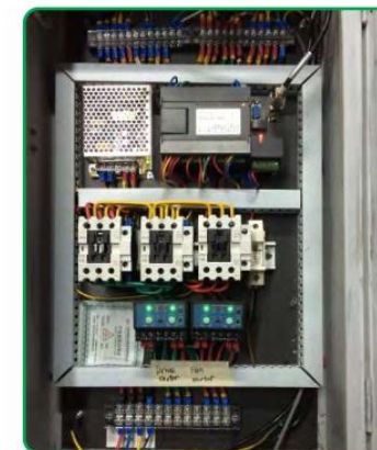
Electric Box 电箱更新
